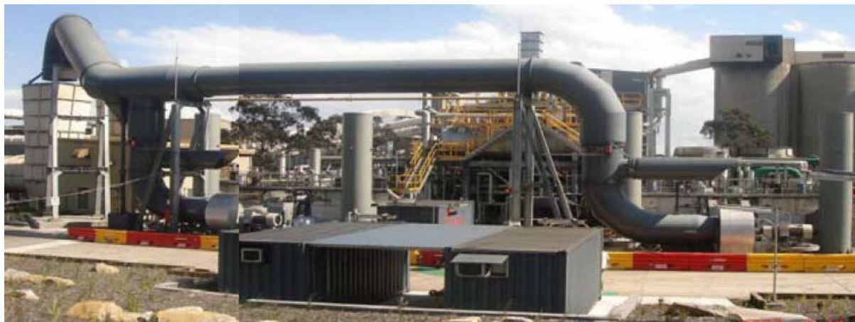
Figure 9: West Cliff Colliery mine ventilation air methane abatement and utilisation plant – WestVAMP
